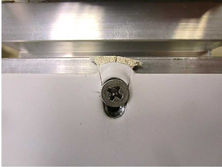
Photo No. 9 Typical Fastener Shear Failure Mode Detail
